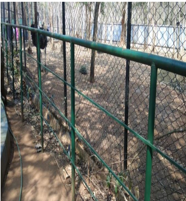
Construction of Protection mesh for visitors in front of Emu and Ostrich birds
