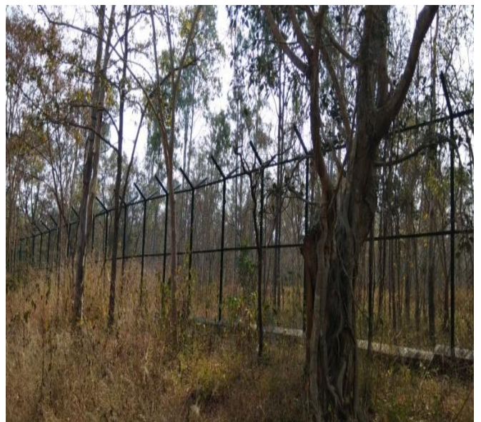
Y angle and chain link mesh painting
